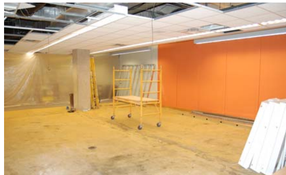
Already gutted and beginning to take a new shape, the Hansen Teen Library Center pictured on Aug. 18.
